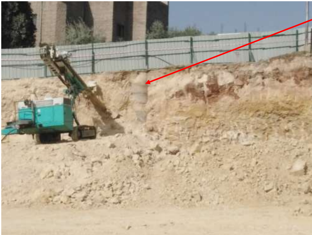
Existing manhole : The Contractor must protect the manhole during the excavation works
