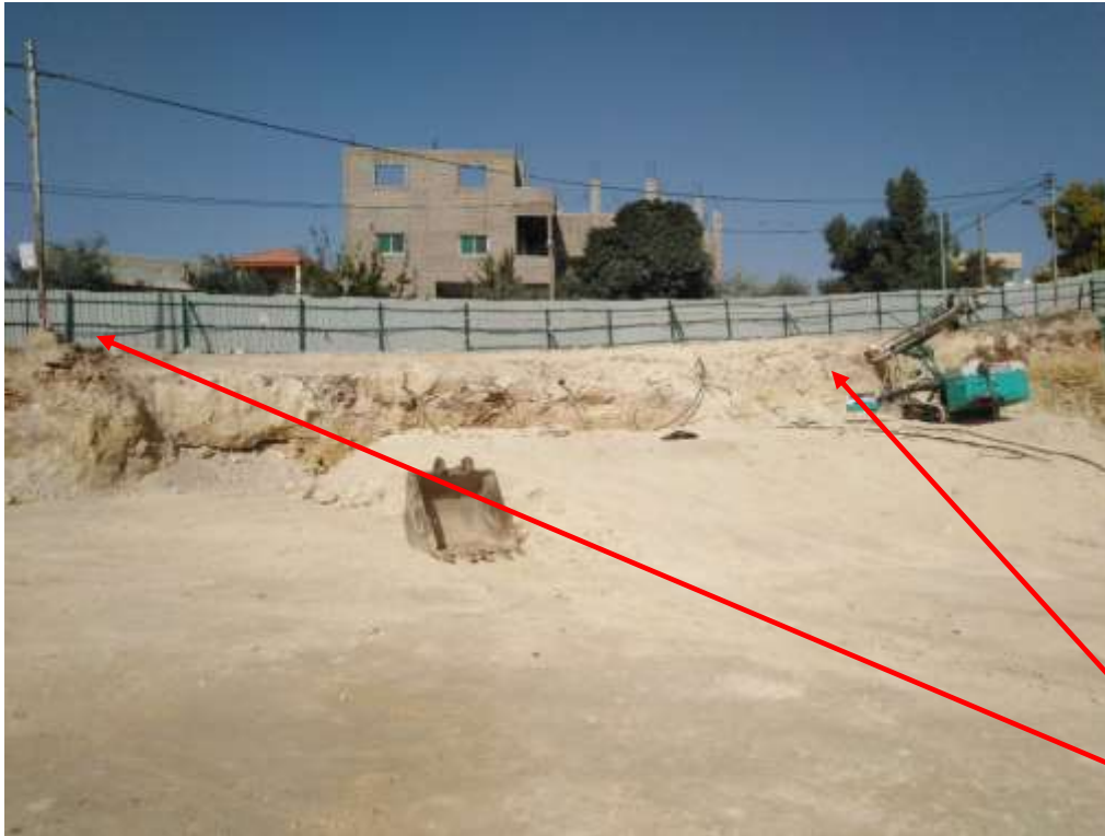
FIGURE #02 & 03: Shoringssystem started to protect the area from soil sliding and protect the electricity poles from falling down
