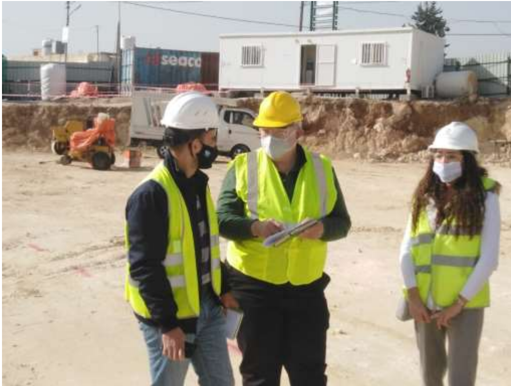
FIGURE #02 & 03: During the site tour of USAID, CMTO, SE and the Contractor to check the drawings and inspect the excavation works and unsafe vertical
