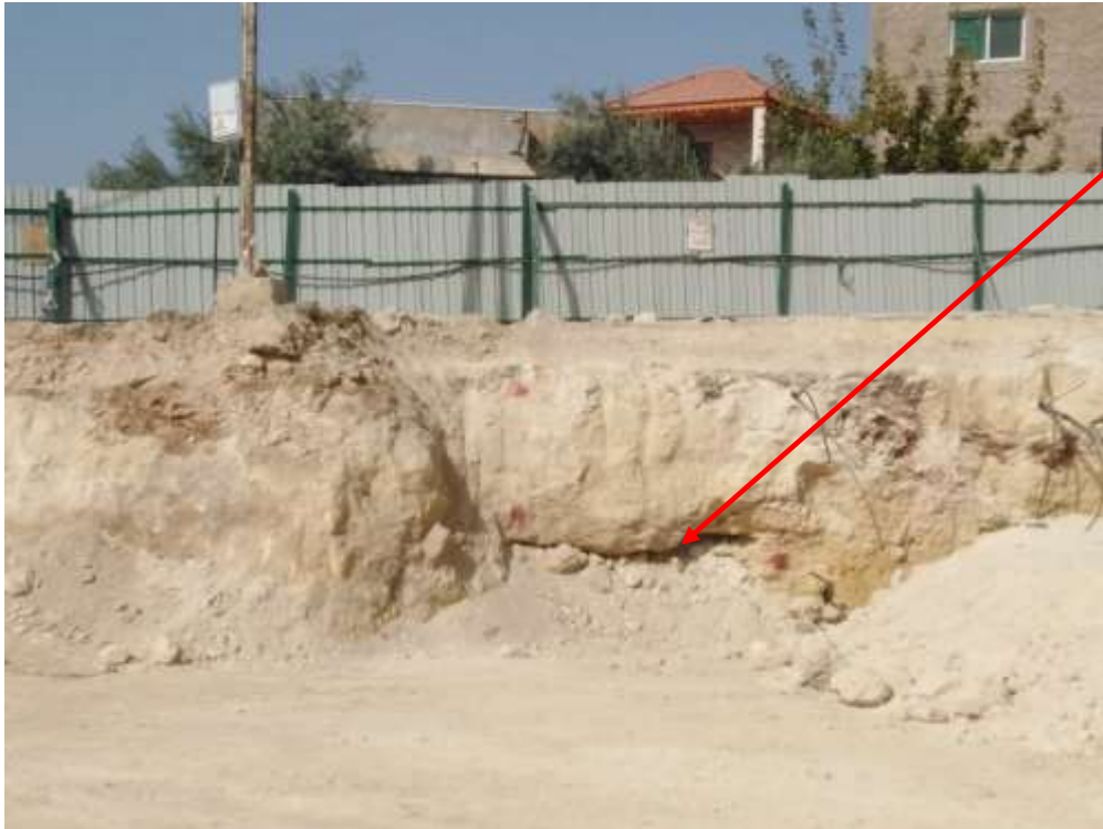
FIGURE #04: This area needs to be checked by Geotechnical lab to determine if it is a cavity or not before starting the construction the retaining walls.
